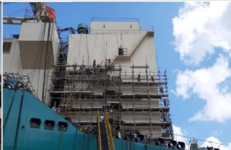
DF Module general view Port side
