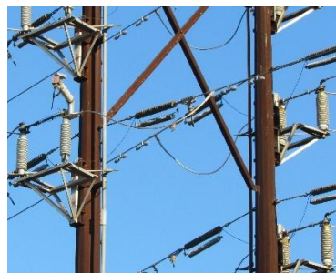
Power Transmission Line
