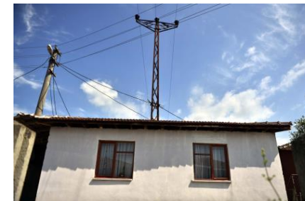
Power Distrubution Lines to the buildings
